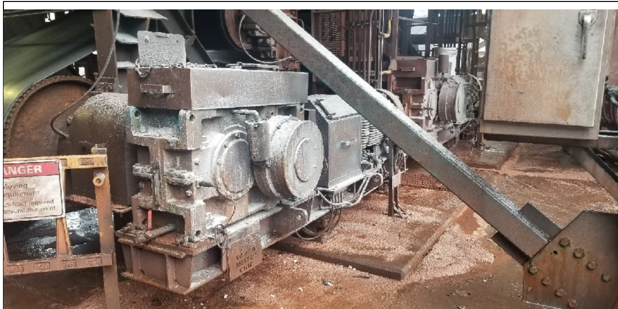
Photo No. 21. Date: 2022-JUN-1 Direction Facing: N/A Description: View of the belt drive motors for Conveyor 8.
