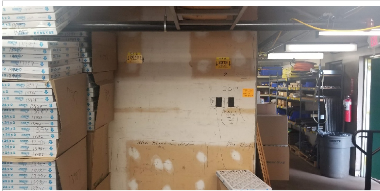
Photo No. 7. Date: 2022-JUN-1 Direction Facing: North Description: View of the drywall panels and exposed asbestos containing drywall joint compounds located in the upper floor of the Old Stores Building.
