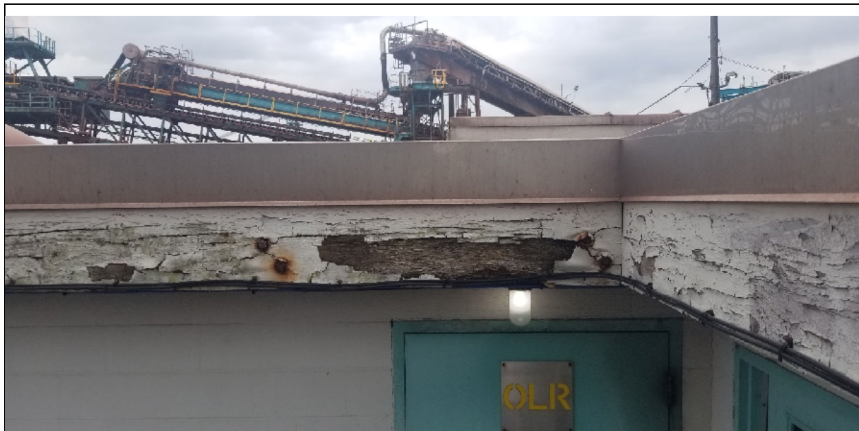
Photo No. 8. Date: 2022-JUN-1 Direction Facing: East Description: L26 – Old Stores Building wood trim, white paint with lead concentration of 1280 mg/kg.
