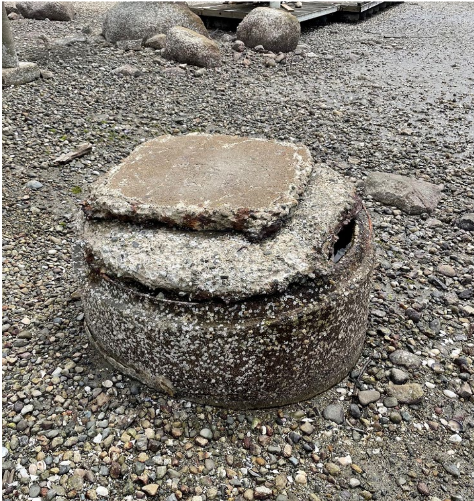
Example of a junction point of the sanitary main along the foreshore
