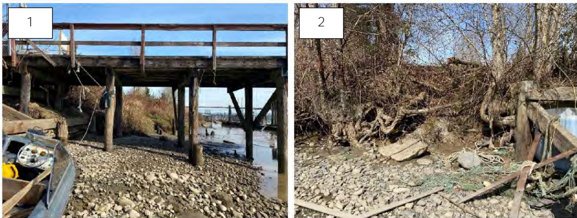
Photographs 1-2. (1) Facing east, looking at the Fraser River foreshore, immediately south of Bonson Road. Erosion was visible and unprotected banks were noted. (2) Facing north, looking at vertical banks and failing riprap (Photographs from NHC, 2022).
