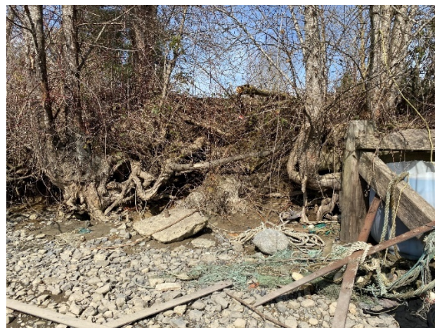
Photo 2. Nearly vertical bank and failing riprap, 30 m downstream from the dock.
