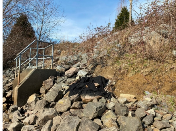
Photo 4. Riprap failure exposing the filter fabric and underlying soil at the existing stormwater outfall location.
