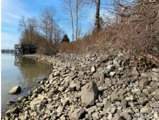
Photo 3. Larger-sized riprap near the existing stormwater outfall. Large rocks in the water suggest signs of failure or loss of stones during placement.
