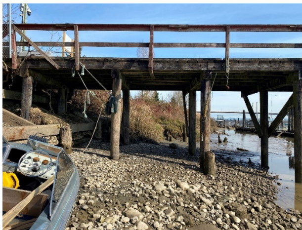
Photo 1. Existing bank protection just at the south of Bonson road. Signs of erosion can be seen in the unprotected bank in the background of the dock.
