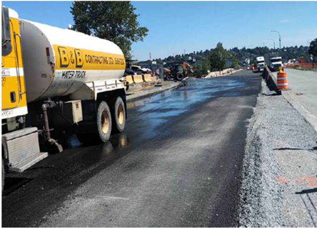
Pictured: Water placement on the road to control dust during construction activities
