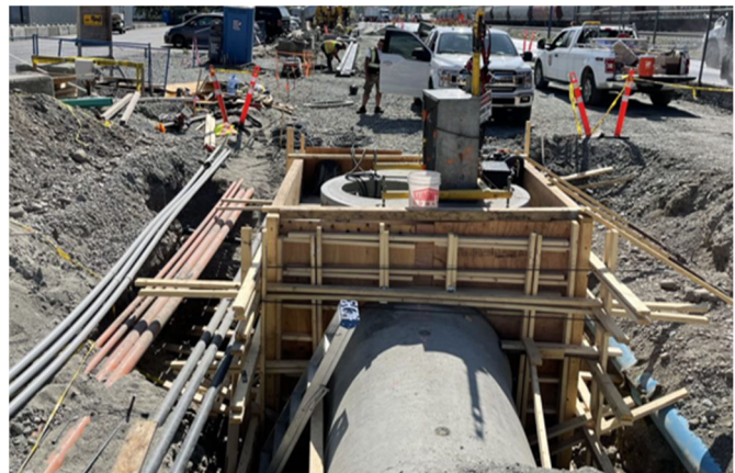
Pictured: Formwork in place for the new manhole that will provide access to the utilities pipe
