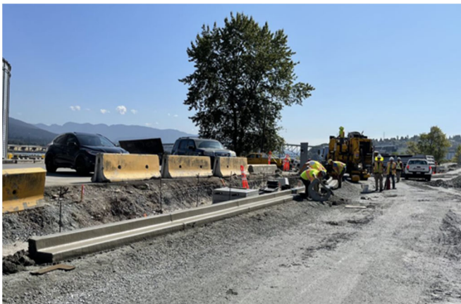
Pictured: Pouring concrete for the road curb and gutter next to Columbia Containers
