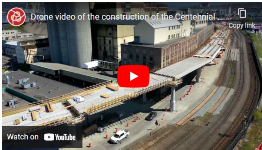
This flyover drone video shows the April 2021 progress of construction activities associated with the new Centennial Road overpass, part of the South Shore Access Project.
