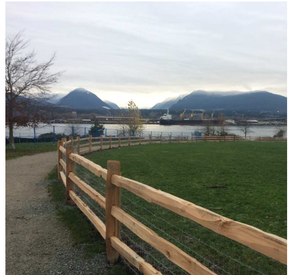
New dog off-leash fencing installed on the west side of the park.
