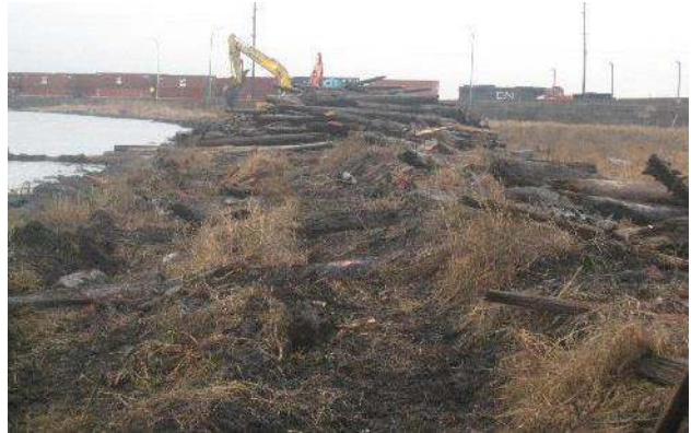
Photo 2. Excavator shifting woody debris towards the load-out area during restoration works (January 2014).
