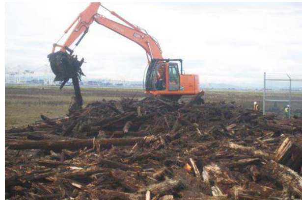
Photo 4. Excavator shifting woody debris toward the load-out area during restoration works (March 2013).
